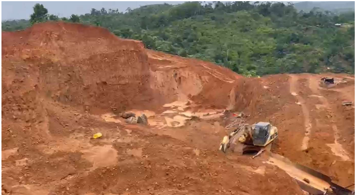
Fig. 131: Grab from video taken on 20 May 2026 showing the state of the abandoned illegal workings at Akoko South. Note the high wall at approximately 18m.
